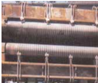
Air mist nozzles fed and installed by means of small and long hydraulic pipes
