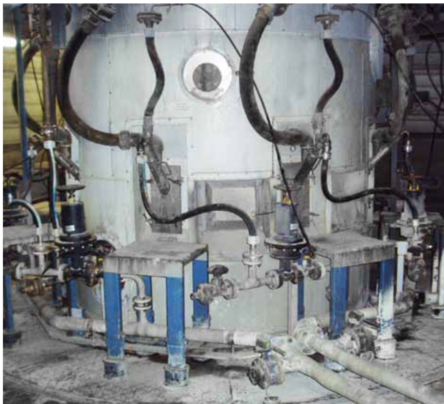
Twin-fluid nozzle lances in an existing system, with tables for the frequently necessary disassembly and cleaning of the nozzle lances
