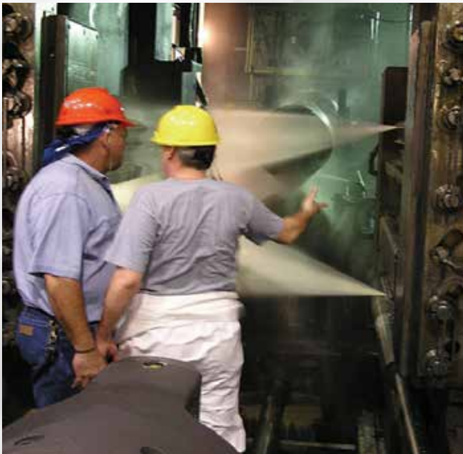
Internal evaluation shows severe contamination inside pneumatic chamber header.
