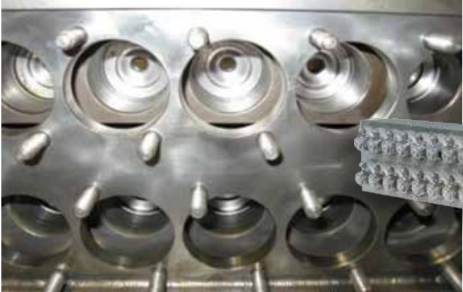
SELECTOSPRAY® header after acid cleaning
