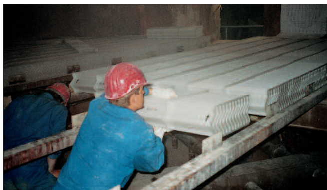
Assembly of the LTV 400, plastic, in a flue-gas desulphurization plant
