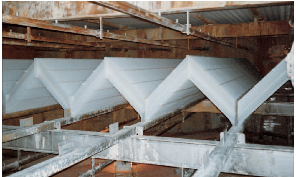
LTV 110.33-B in a wash tower
