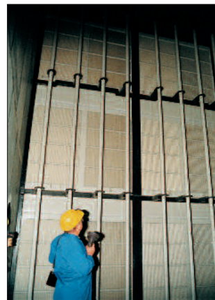
Installed LTH 100 in a flue-gas desulphurization plant
