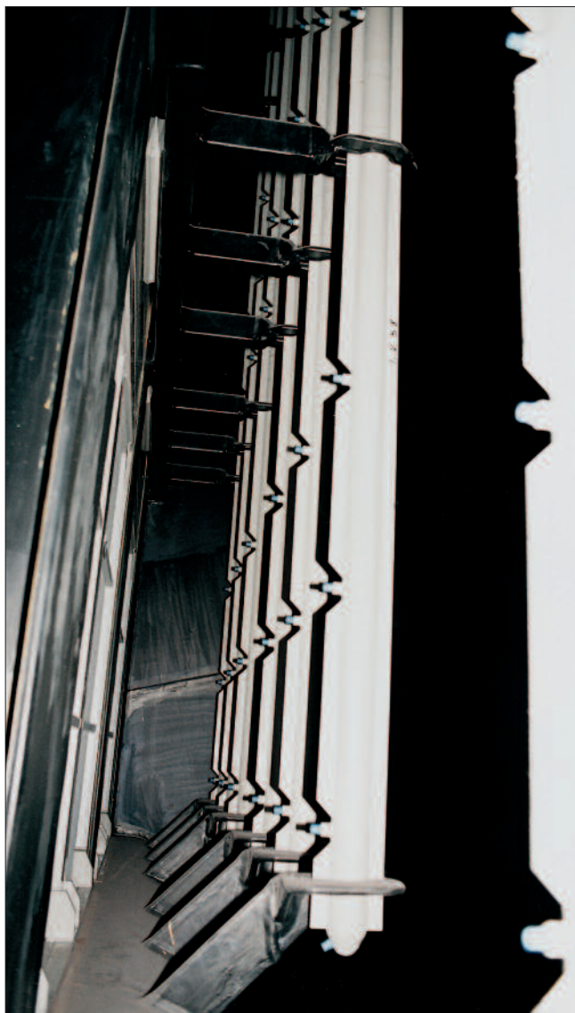
Nozzle spray system
