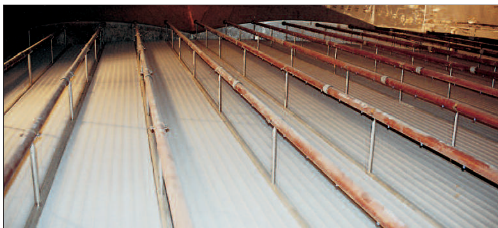
LTV 271 as a fine separator in a flue-gas desulphurization plant
